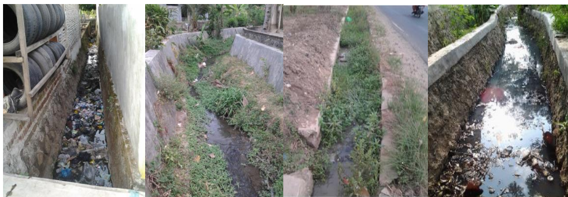
Figure 2. Drainage Canals Condition at Gedongtataan Source: Field Observation (2015)
